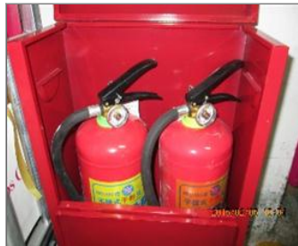
Photo of the inside of the main production hall Fire extinguisher (3).JPG
