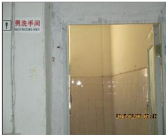
Photo of the sanitary facilities Lavatory (2).JPG
