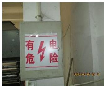
Photo of the inside of the main production hall Electric switch box.JPG
