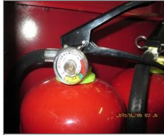
Photo of the inside of the main production hall Fire extinguisher (2).JPG
