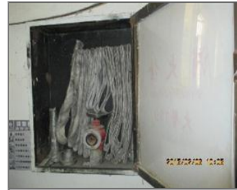
Photo of the inside of the main production hall Fire hydrant (2).JPG
