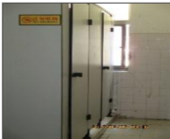
Photo of the sanitary facilities Lavatory.JPG
